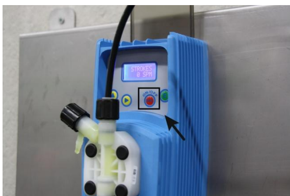
Figure 5: Switching the pump on
