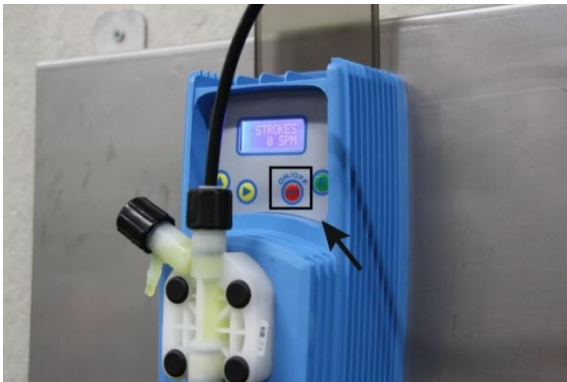
Figure 5: Switching the pump on
